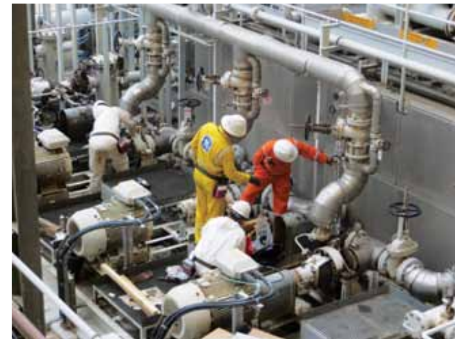
The LNG Train 6 shutdown project provided a perfect example of Qatargas employees and external contractors doing what they do best: working as a team, while showing mutual and genuine and mutual care for people and facilities.
